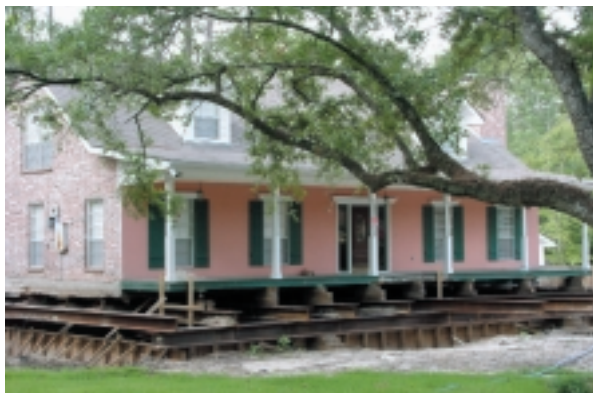
Raising a house can be a costly option for the homeowner. This slab-on-grade home in St. Tammany Parish, Louisiana, was raised at a total cost of approximately $150,000. A matching grant from FEMA's Pre-Disaster Mitigation program pays 75% of the expense to raise a home, with the homeowner bearing the remaining 25% of the cost.
